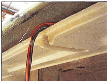
Counter-moulded deck/Electrical wiring
